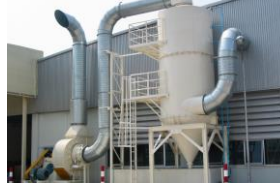
WET SCRUBBER SYSTEM
