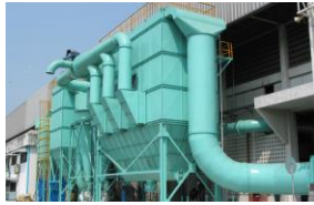
DUST COLLECTOR SYSTEM
